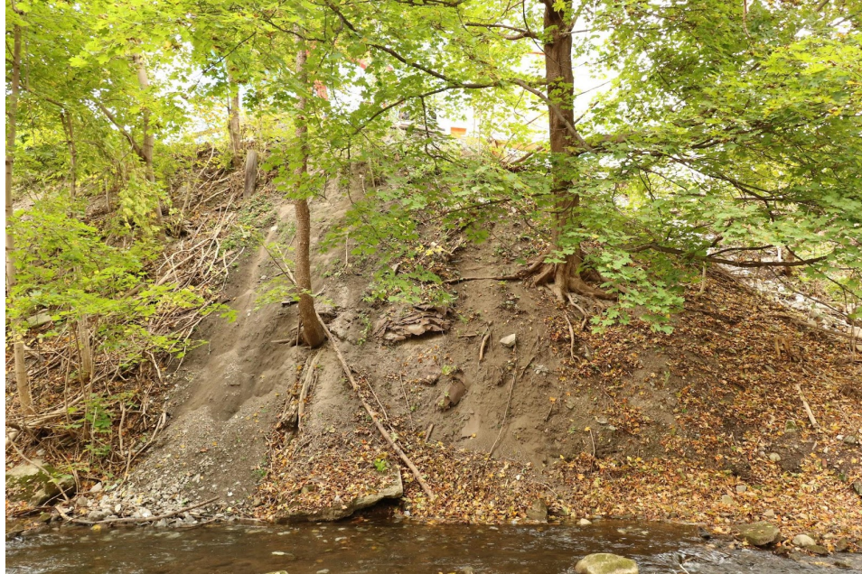
Figure 5. Site of Predicted Landslide
