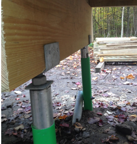
Figure 18: Close-up of pile system: Square plate tops the hollow pile, round pile below anchors the bride (Photo property of Ken Allard)
