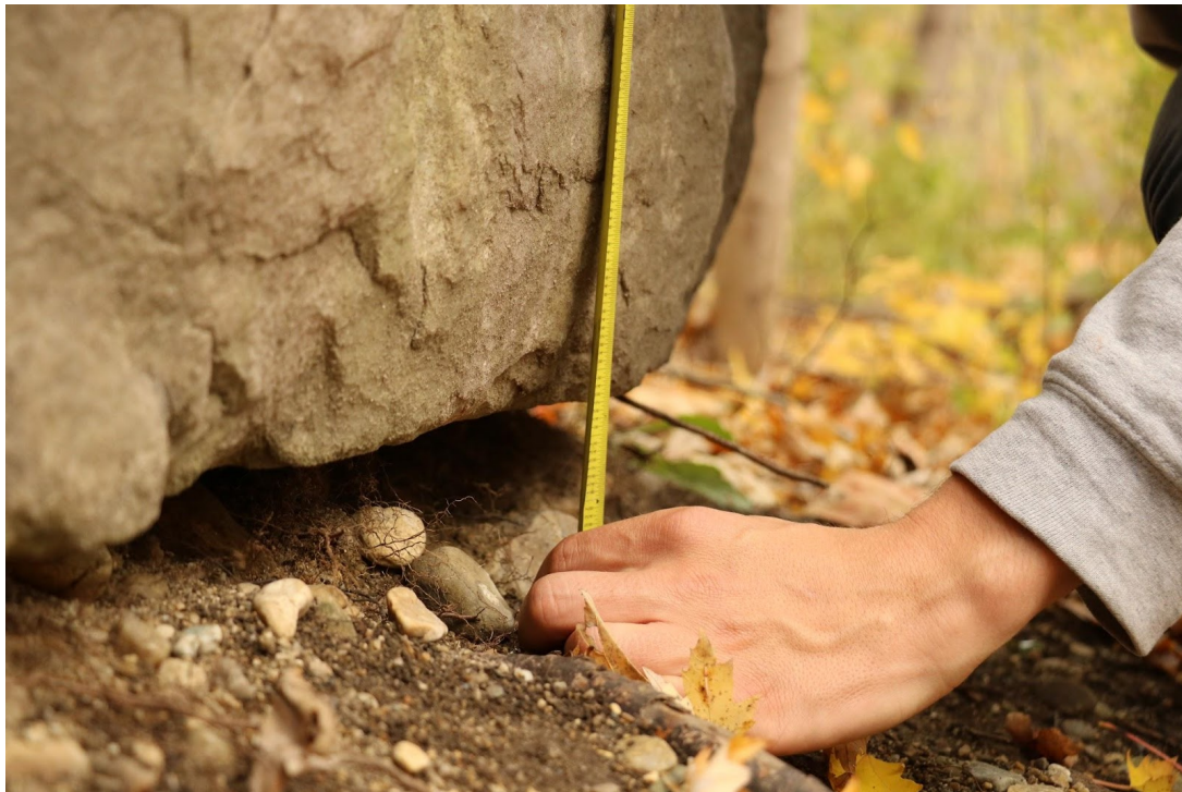
Figure 5: Scour present on the current abutments
