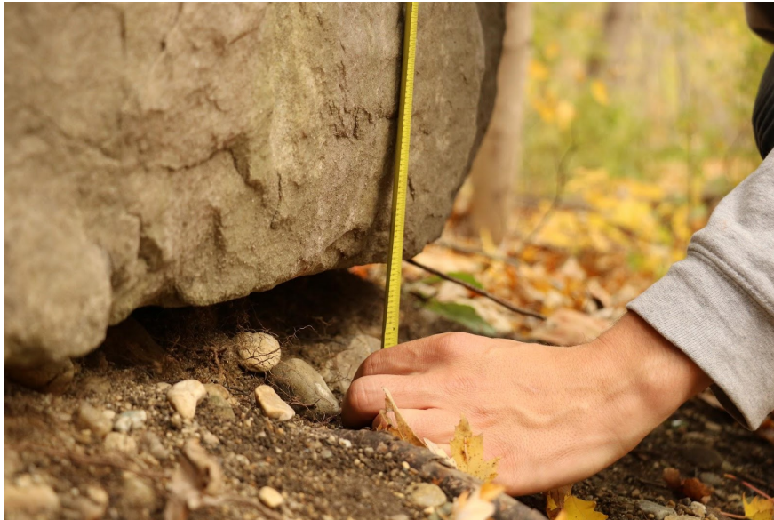
Figure 10: Scour on the Current Abutment
