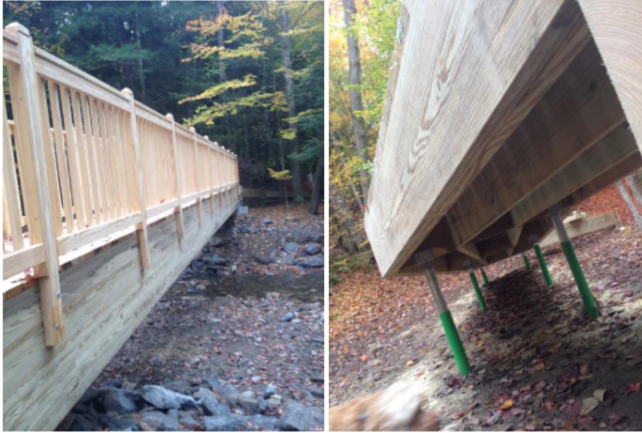
Figure 13: Hapgood Pond “floating” bridge structure (left) and adjustable sleeve piles supporting the structure (right) (Photo property of Ken Allard)
