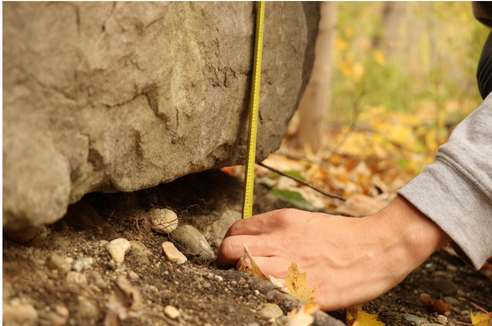
Figure 19: Existing Scour on Abutments
