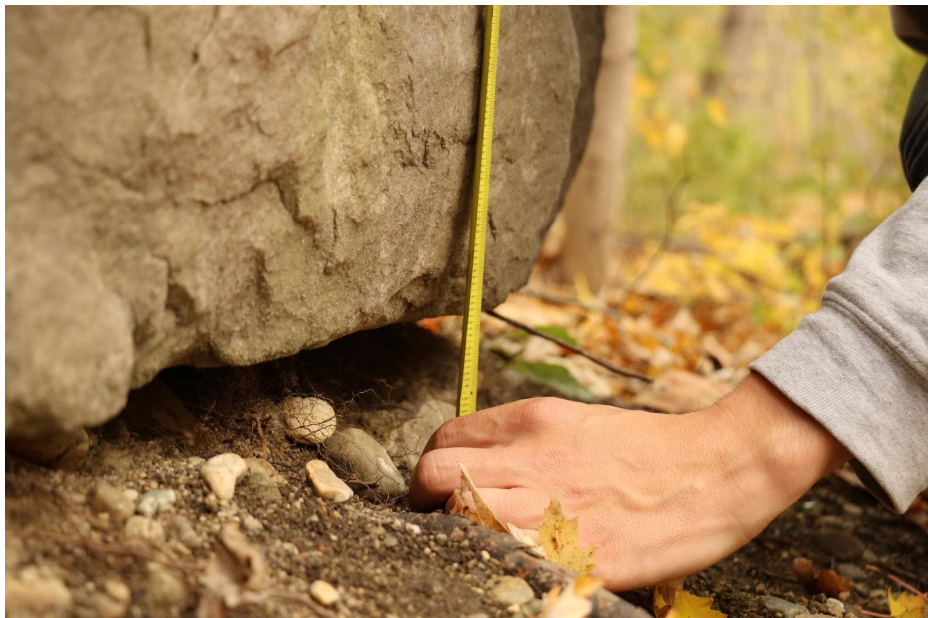
Figure 4. Current Scour on Existing Abutments
