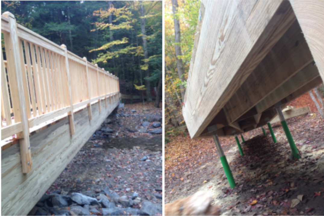
Figure 16: Hapgood Pond replacement, “floating” bridge structure (left) and adjustable sleeve piles supporting the structure (right) (Photo property of Ken Allard)
