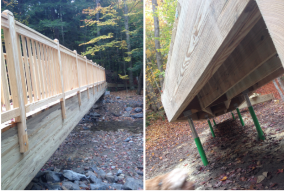
Figure 7: Hapgood Pond “floating” bridge structure (left) and adjustable sleeve piles supporting the structure (right) (Photo property of Ken Allard)
